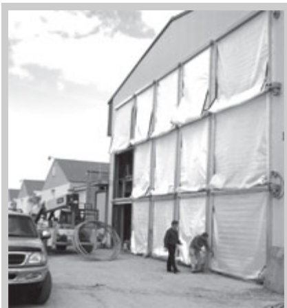
Dave Andrews and Tom Beachler checking the ventilation system at Kreider's Farm.
